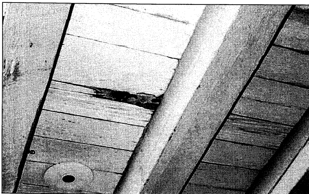
View of damage to interior ceiling
