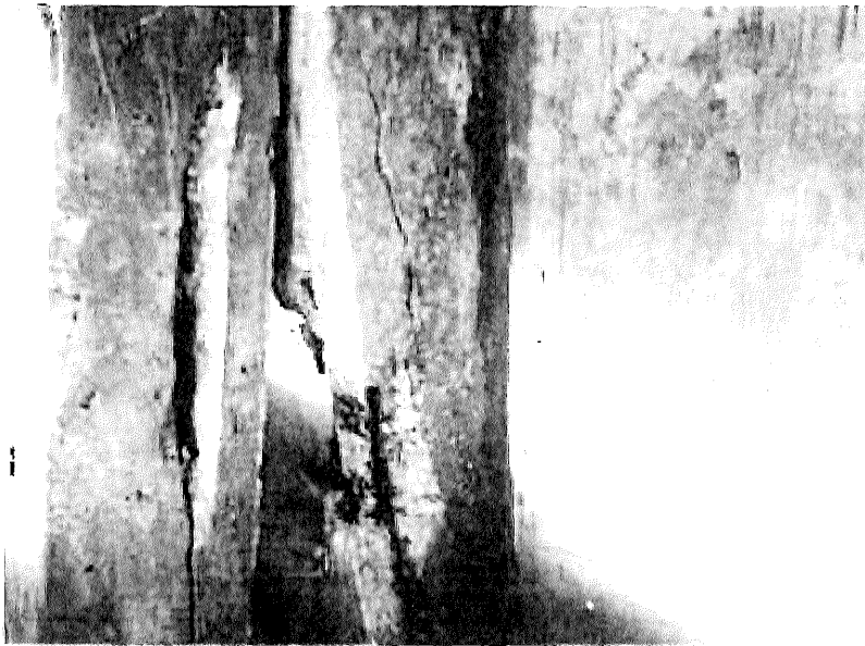
Photos from structural report
