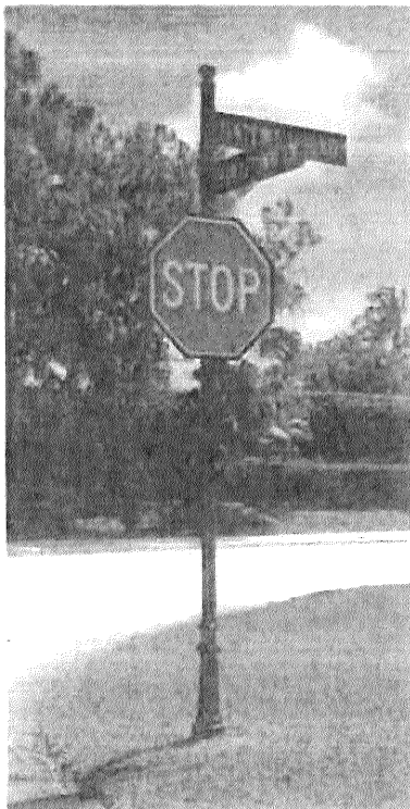
REGULATORY "R1-1:" Sign #9 NOT in compliance with MUTCD
