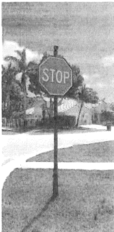
REGULATORY "R1-1:" Sign #13 NOT in compliance with MUTCD
